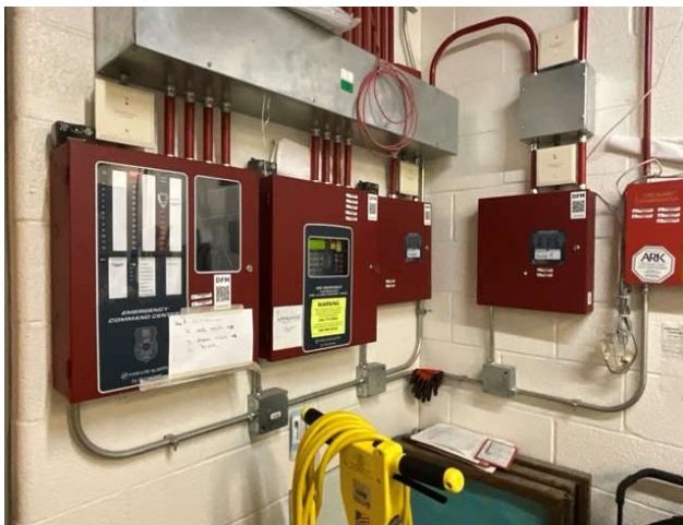
21 - FIRE ALARM PANEL
